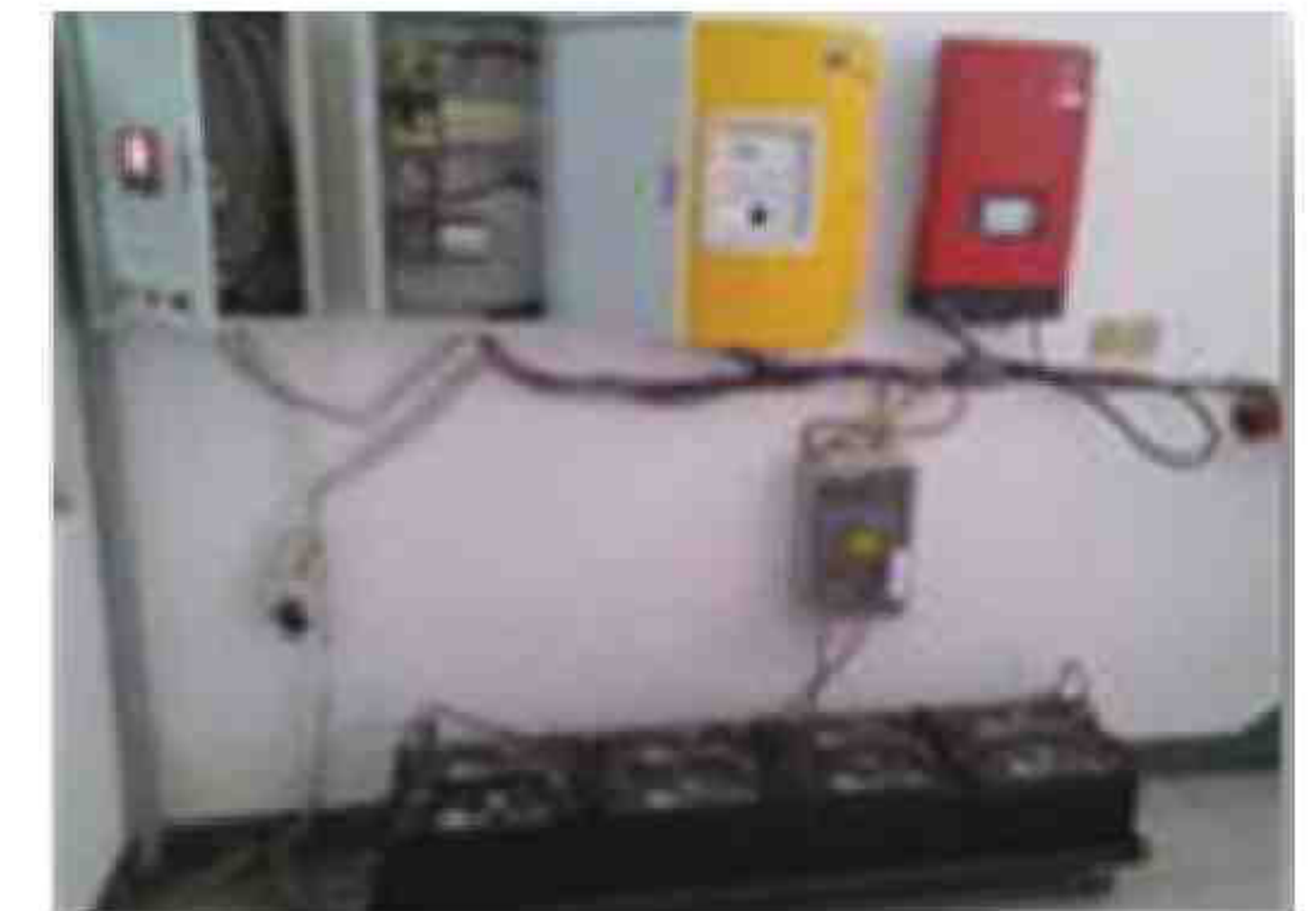
Smart Microgrid, 5kWp Hybrid Inverter, 1kWp PV System, 9.6kWh Battery System
